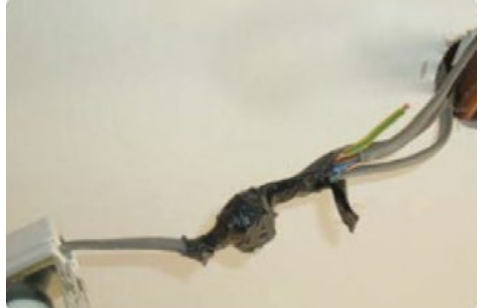
Unsatisfactory connections to a downlighter, requiring a Code C2.
