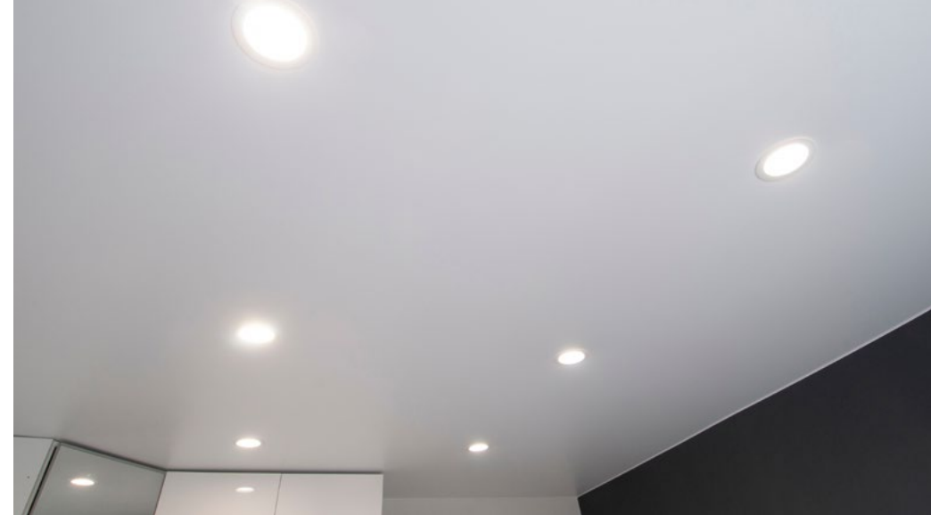
Enclosed ceiling lights
