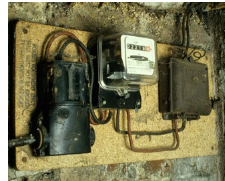
Fusebox with a wooden back
