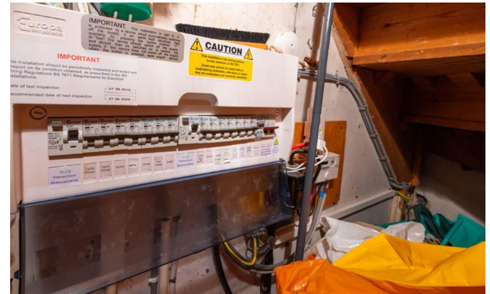
Don't store combustible materials close to electrical equipment
