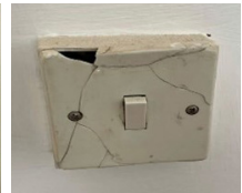
Damaged light switch.
