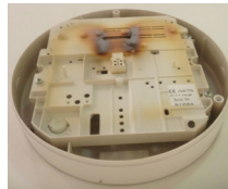
Overheated light fitting (wrong lamp used).
