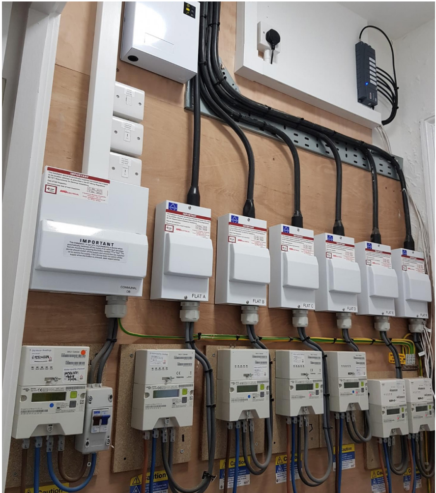
Figure A1: Example of group metering at the electrical intake position/origin. Photo courtesy of AMD Electrical
