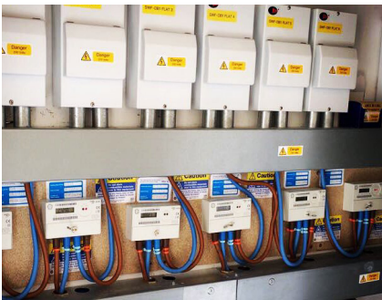
Image courtesy of MAK Electrical Services.
