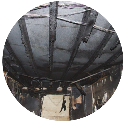
Result of an eight minute fire on lightweight joists (Courtesy of Manchester City Council - Building Control)
