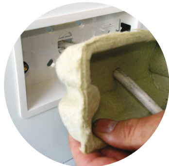
Intumescent pad being installed in a dry lining box (Photo courtesy of Knauf Drywall)
