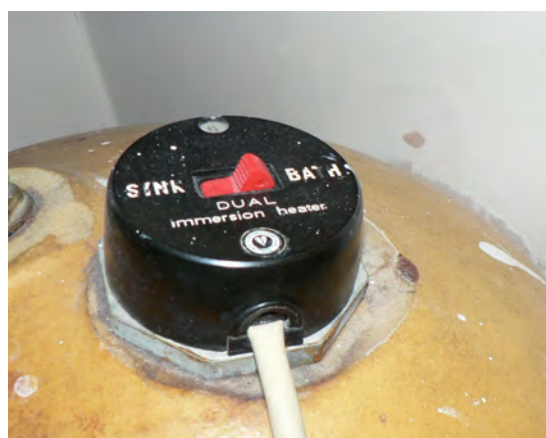
Older immersion heater without thermal cut-out
