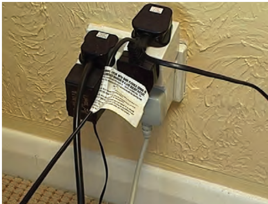
Inadequate provision of socket-outlets
