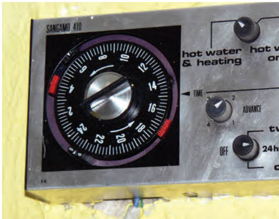
Cable sheath not taken inside metallic enclosure
