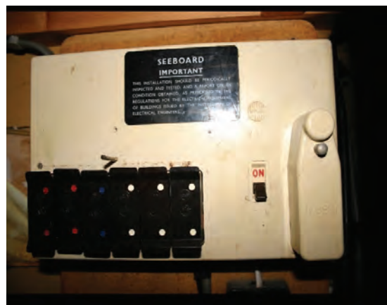
Consumer units having rewirable fuses can continue to provide satisfactory service (Cover removed for illustrative purposes)
