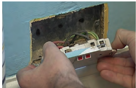
Socket-outlet with broken face plate
