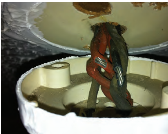
Crumbling vulcanised rubber insulation
