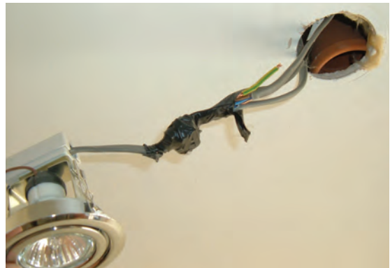
Unsatisfactory connection to a downlighter
