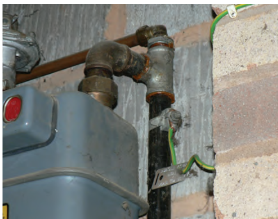
Main bonding connection not made before branch pipework
