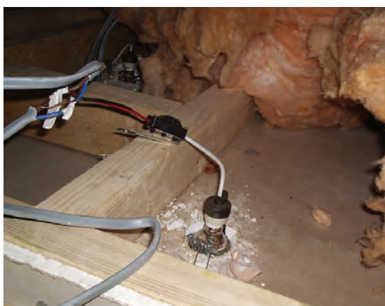
Unsatisfactory electrical connections
